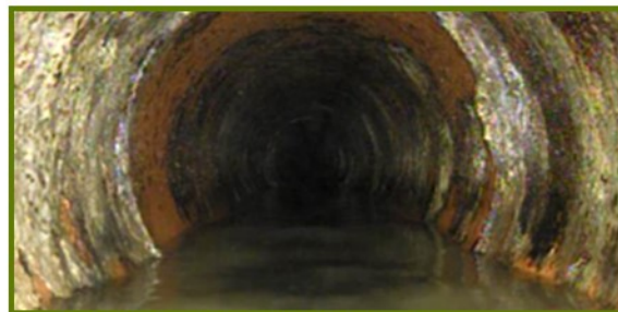
CCTV view of grease lined sewer pipe
