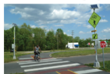
User-activated flashing sign (Rectangular Rapid Flashing Beacon)
