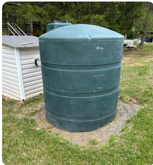
Storage Water Tank
