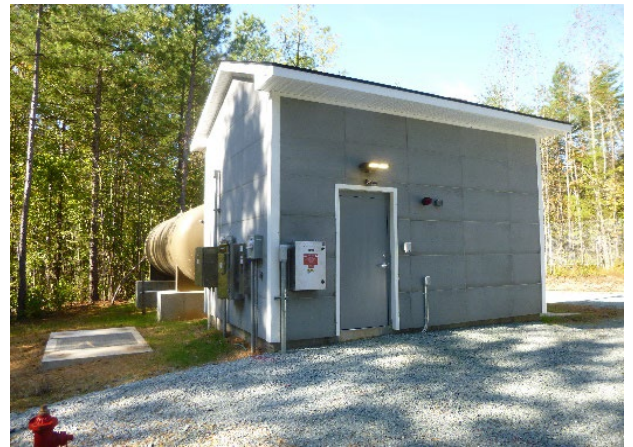
Rougemont Well House and Site Water System Number NC4032018
